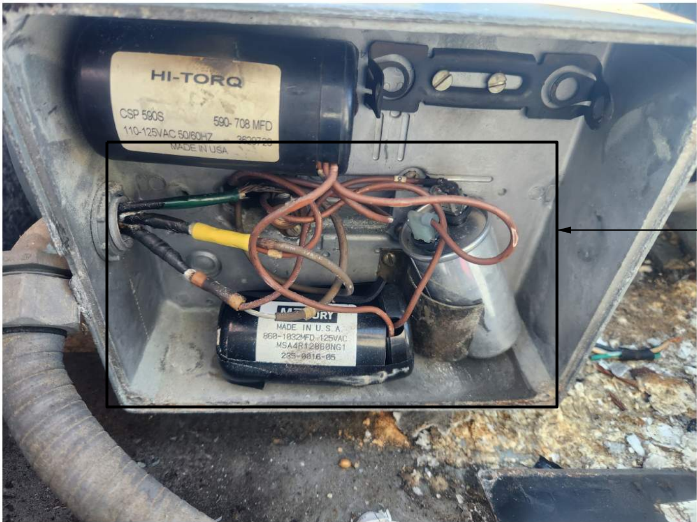
BURNT CONNECTOR ON HPU CAPACITOR
