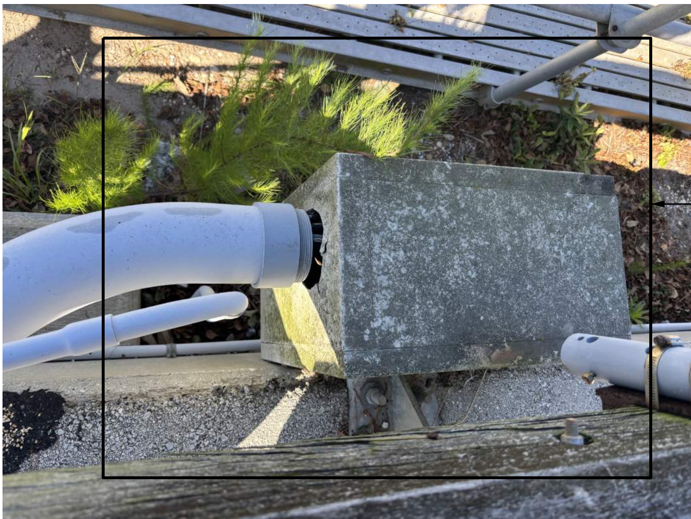
DAMAGED CONDUIT FITTING FOR FIBERGLASS JUNCTION BOX
