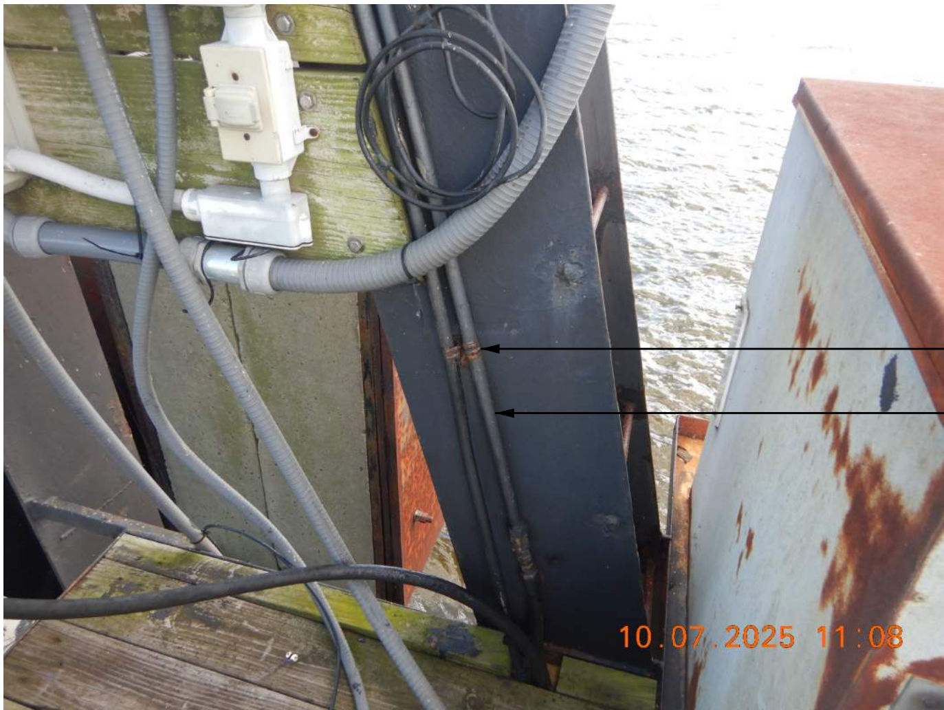
CORRODED TUBING SUPPORTS
