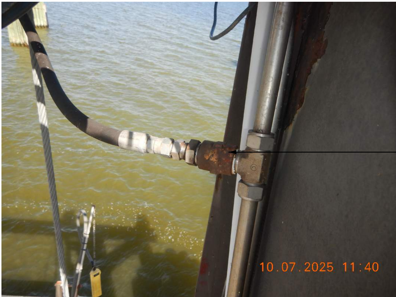
CORRODED HYDRAULIC FITTINGS
