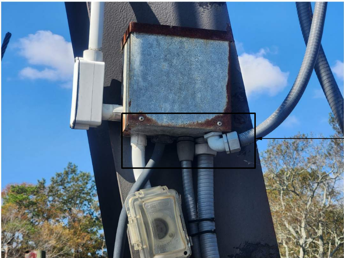
FLEXIBLE CONDUIT FITTING LOOSE ON LIGHTING JUNCTION BOX
