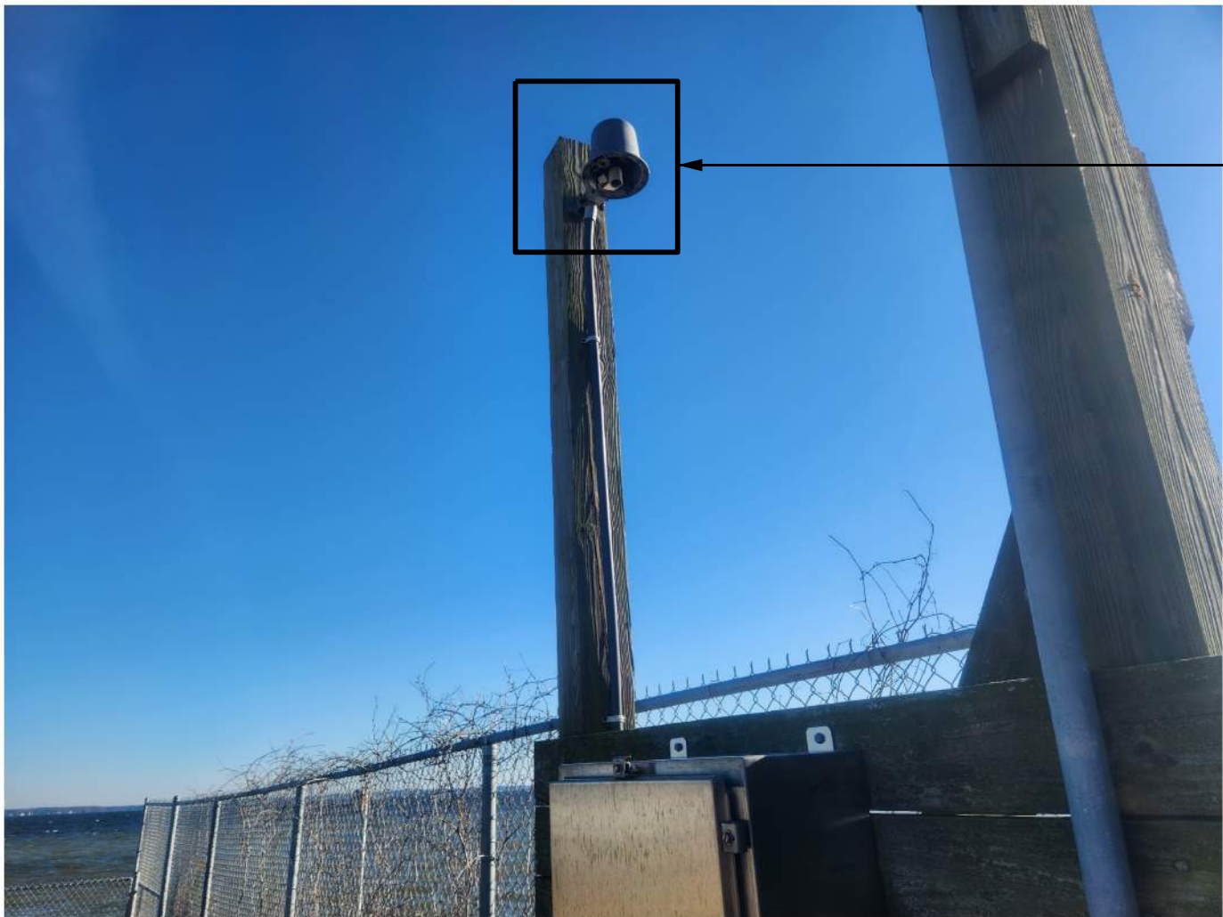
UTILITY PEDESTAL BROKEN LIGHT FIXTURE
