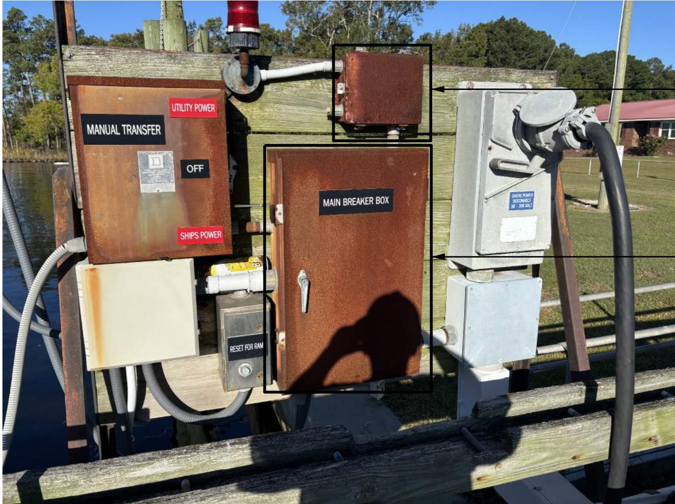
BAYVIEW ELECTRICAL PEDESTAL
