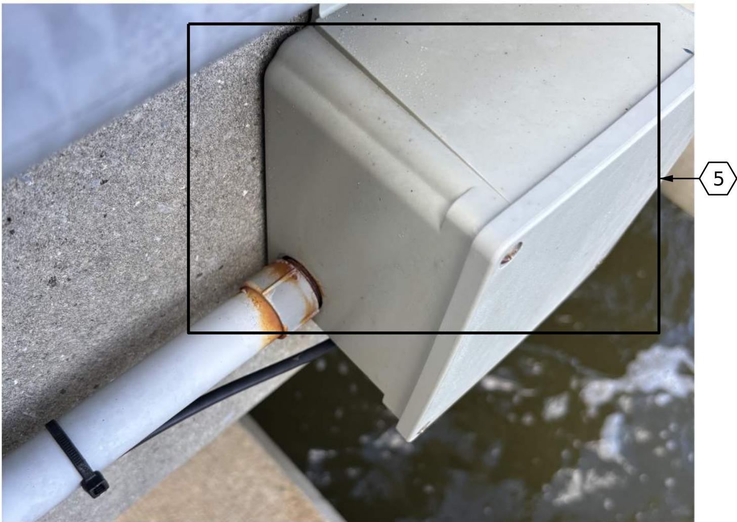
EAST PROFILE RAMP JUNCTION BOX BROKEN OFF CONDUIT
