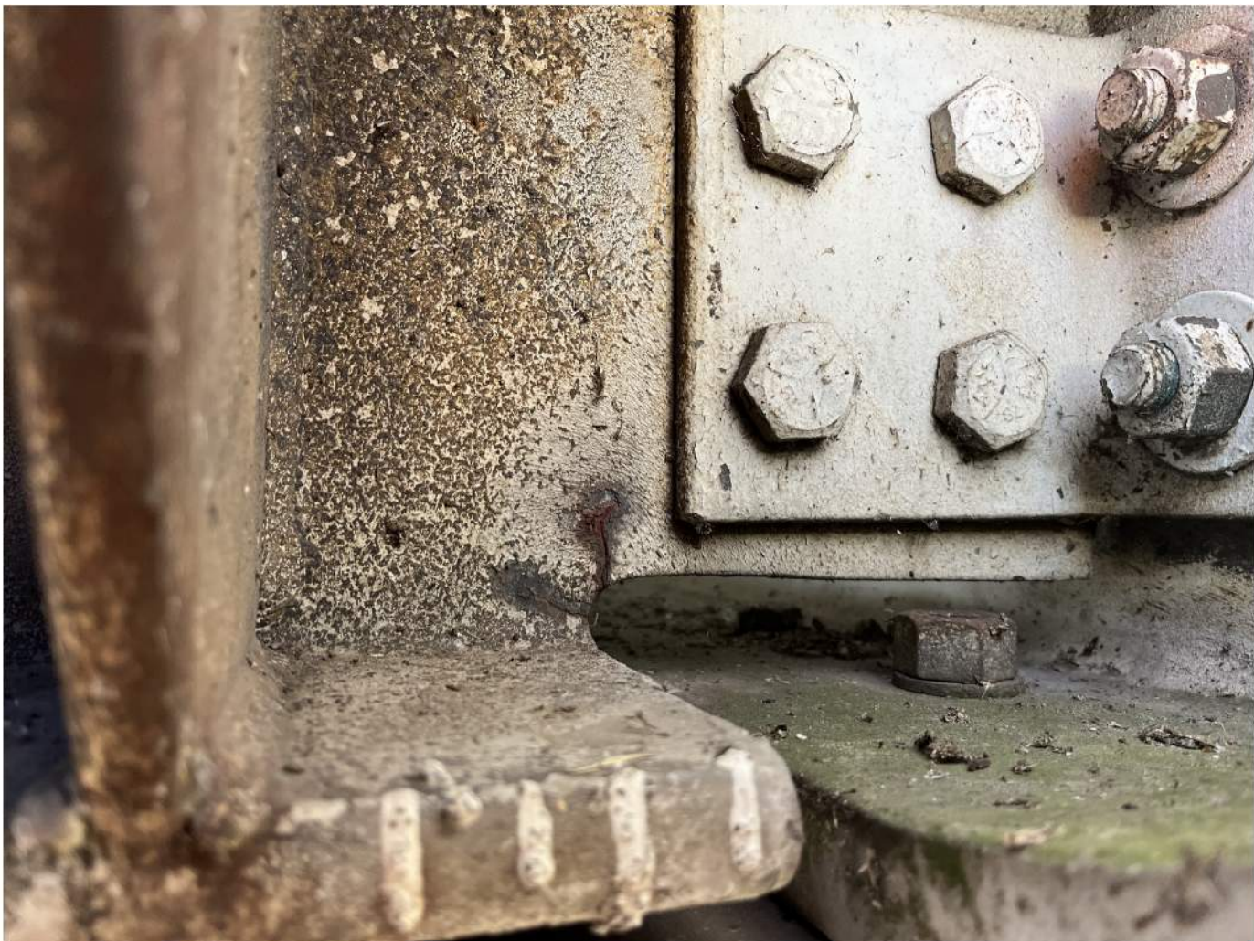
NORTH FACE OF FLOORBEAM 11 AT GIRDER 1
