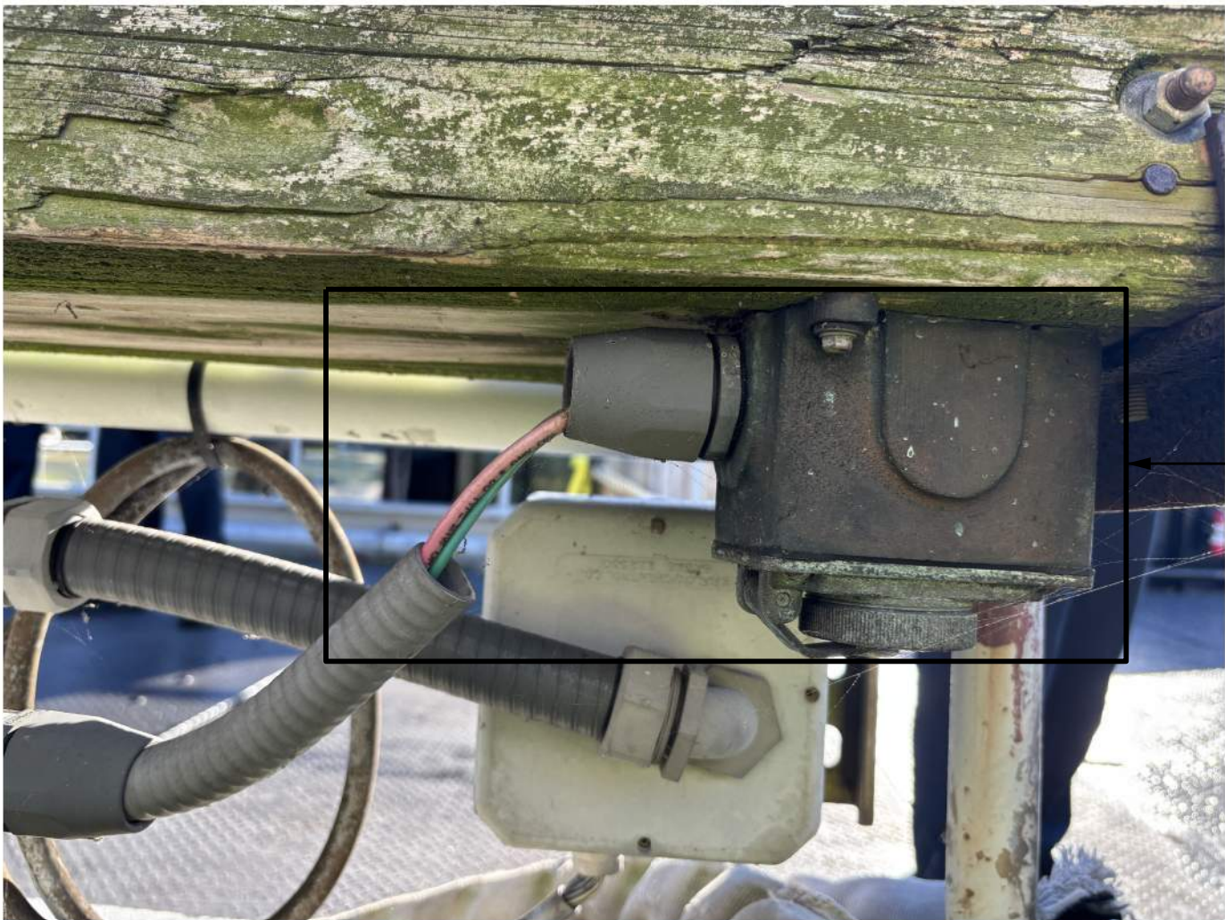
FLEXIBLE CONDUIT DISCONNECTED FROM TWIST-LOCK MARINE RECEPTACLE
