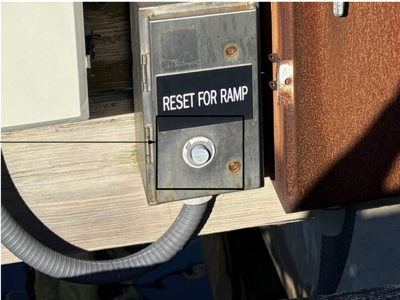
FAILED PROTECTIVE COVER SEAL ON RESET PUSHBUTTON
