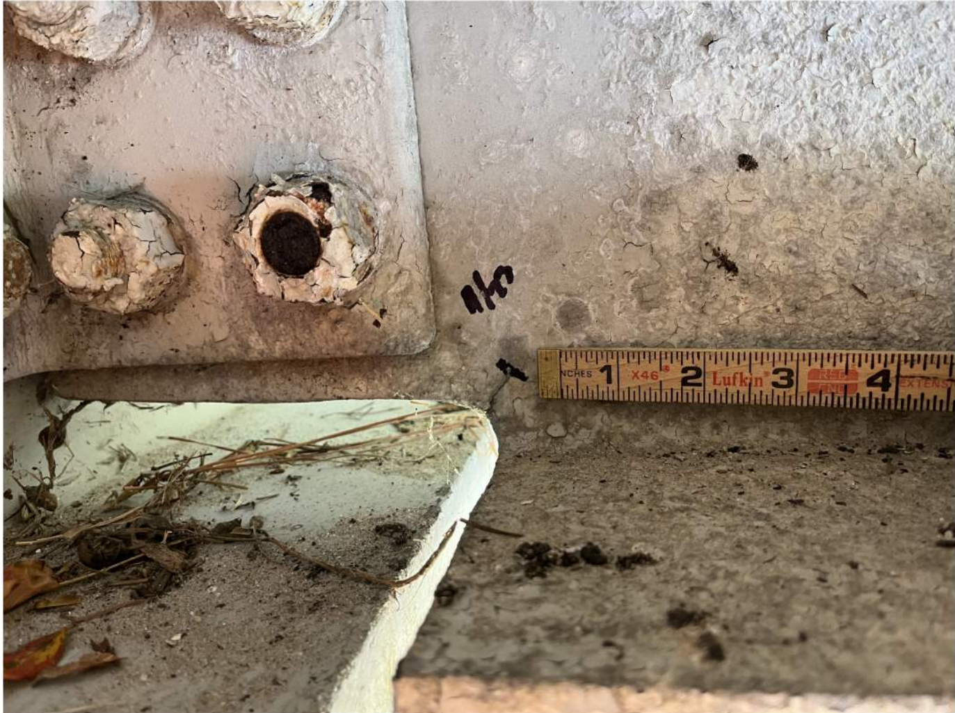
NORTH FACE OF FLOORBEAM 9 AT GIRDER 2
