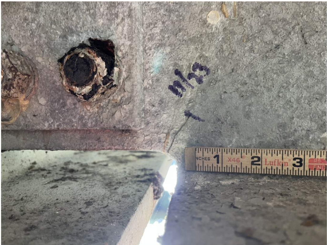
NORTH FACE OF FLOORBEAM 9 AT GIRDER 2
