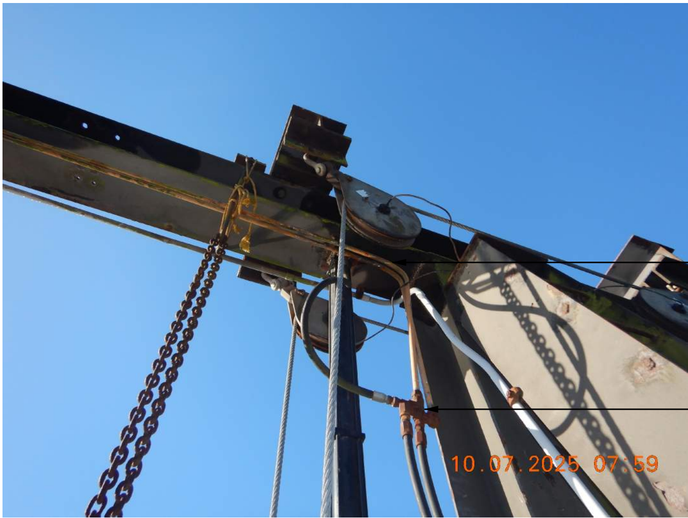
CORRODED HYDRAULIC FITTINGS
