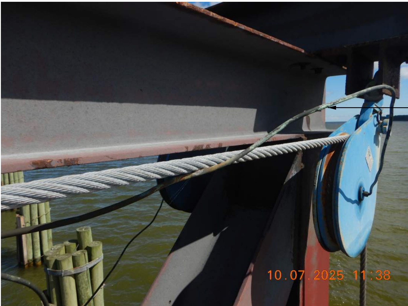
ERRANT GREASE LINE
