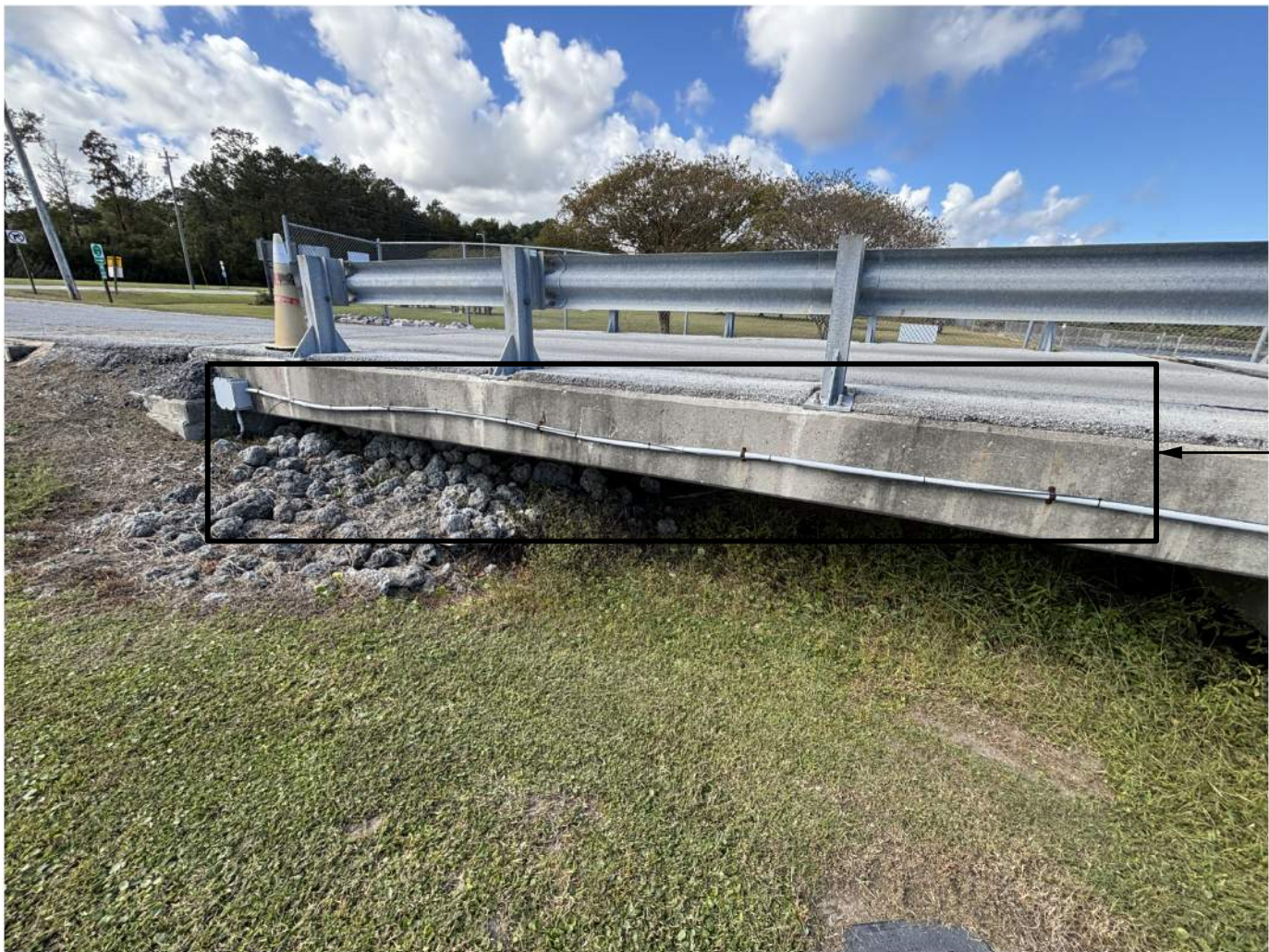
EAST RAMP PROFILE CONDUIT SUPPORTS
