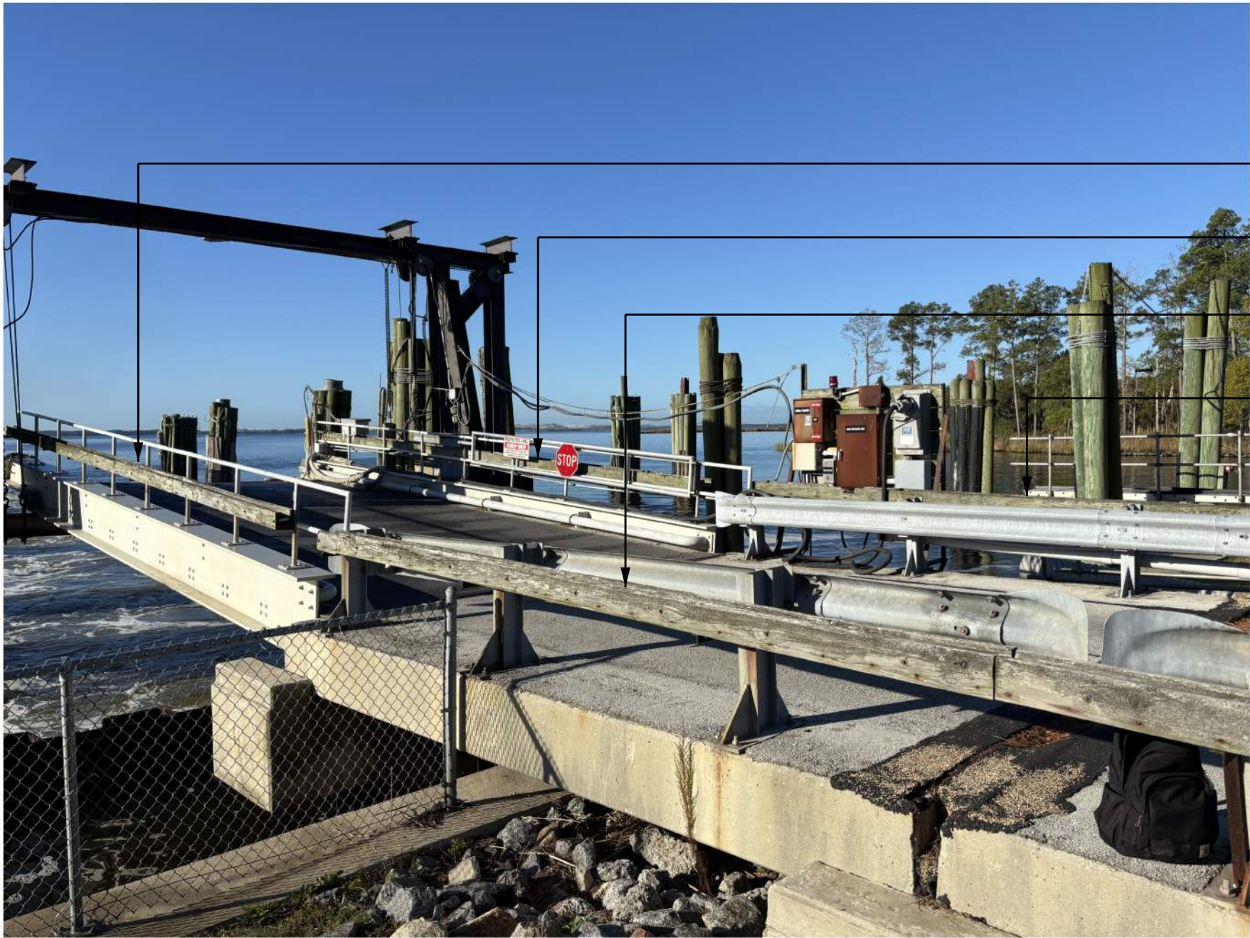
CORRODED CONDUIT SUPPORT ATTACHED TO RACEWAY
